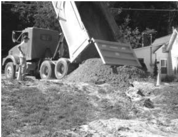
Heavy rains required repairs to the bike trail at Fair Park on Crystal Ave. this fall.
