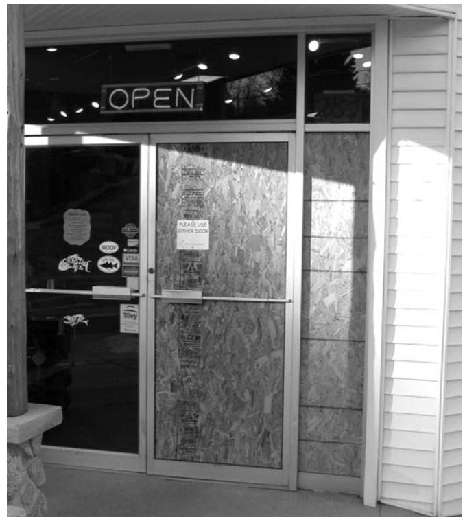
Glass damage from break in at Five Corners
